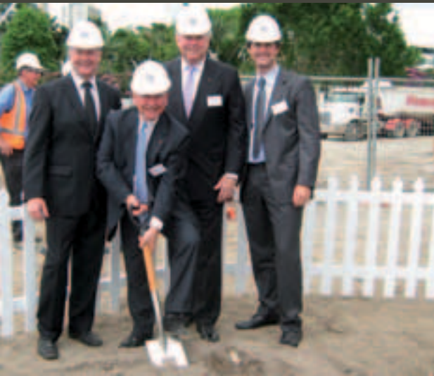
ABC Chairman Maurice Newman turns the first sod on the site of the ABC's new Brisbane premises accompanied by (l-r) Queensland State Director Mike McGowan, Queensland Symphony Orchestra CEO Patrick Pickett and Architect Richard Kirk. Construction of the facility, located at South Bank in the arts and cultural centre of Brisbane, began in May 2010.
