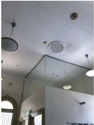
Figure 61: Later front office fitout with early timber-panelled ceiling and ceiling rose above.
