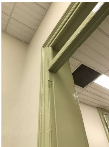
Figure 79: Some doorways indicate earlier door leaf hinge connections, noting early highlight and later false ceiling above.
