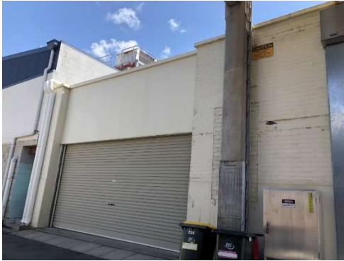
Figure 48: View of the rear elevation showing garage door opening to the western side of the elevated substation.
