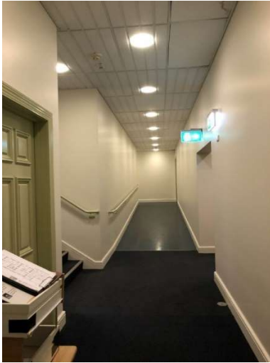
Figure 89: View looking southeast towards the ramp close to the entry into the garage.
