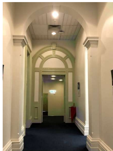
Figure 80: Archways over the end portion of the hallway, noting surrounding pilasters, joinery and moulded skirting and later false ceiling above.
