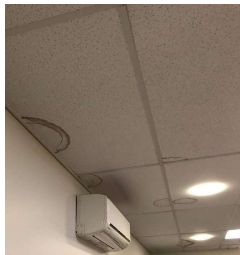
Figure 58: Damaged later ceiling in the existing staff room.
