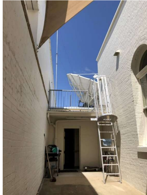
Figure 45: Roof access from the driveway on the south east side of the site.
