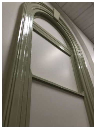
Figure 82: Window with timber frame and infilled panels located within the TV edit room.
