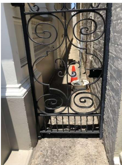
Figure 42: Wrought iron gate at the north-western corner of the front façade connected to the neighbouring property.
