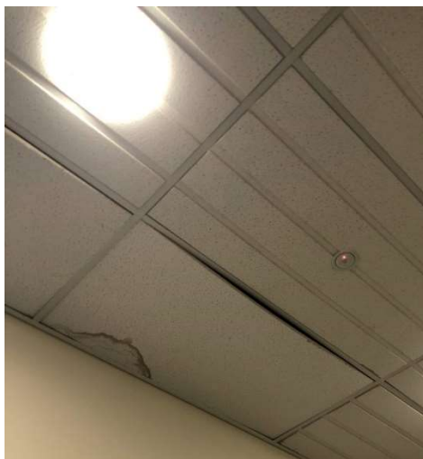
Figure 57: Damaged later suspended ceiling panel.
