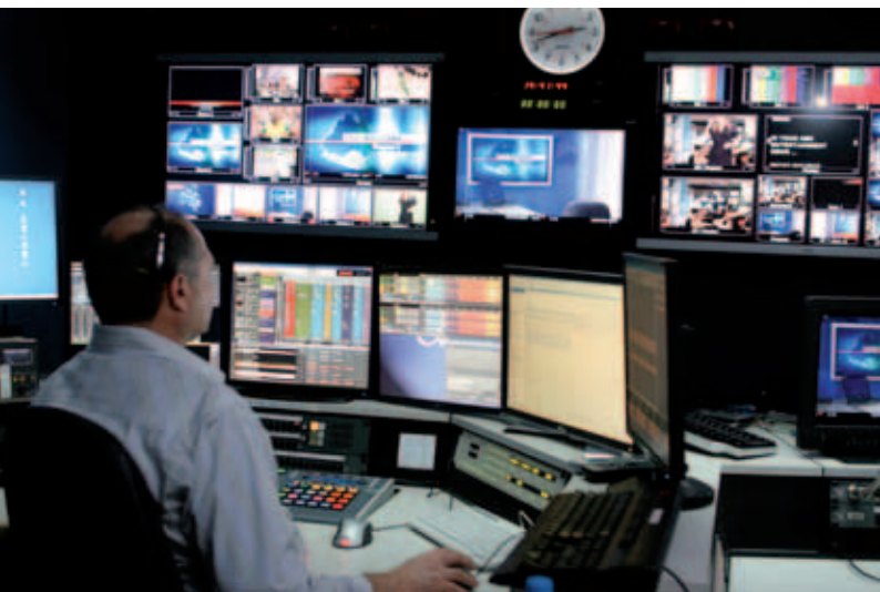
Inside a control room operating with the new Ignite studio automation system.
