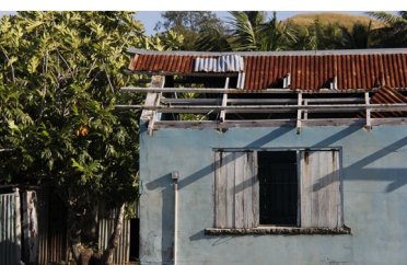
Damaged building in the Yasawa Islands in Fiji. Image credit: Fred Hooper, ABC International Development.
