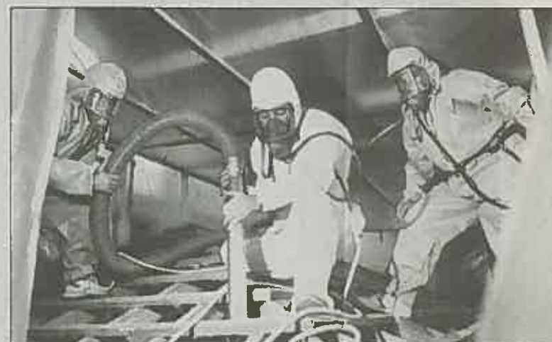
SERIOUS STUFF: Students at Bruce TAFE training in 1990 for a certificate course in asbestos removal, funded by contractors and the ACT Administration branch.
